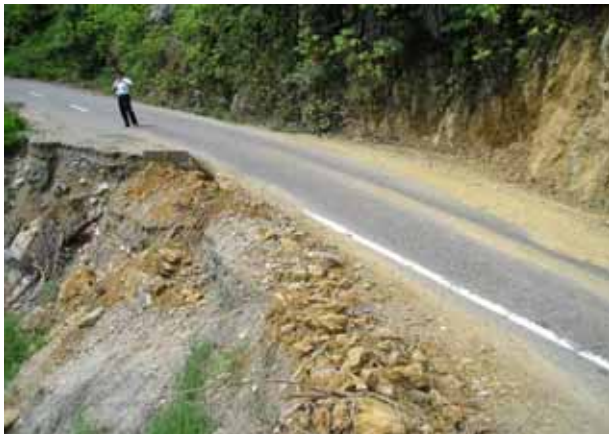
20.8 km from Kluet Utara . Half of the road is damaged and it has a cliff on one side.
