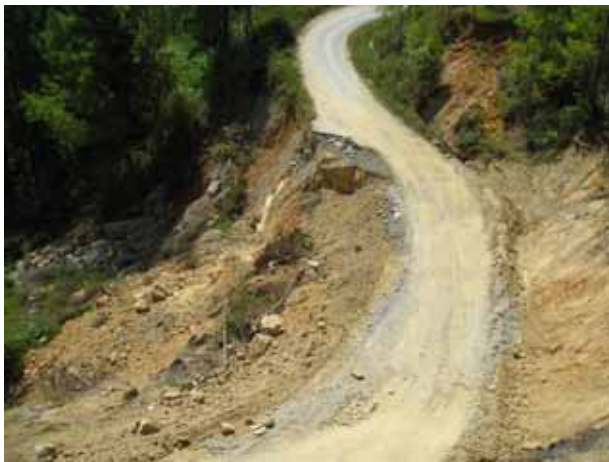
Landslide at the old road which no longer impassable
