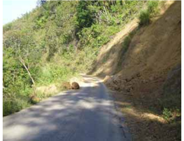
Landslide road on one side and a cliff on the other side.
