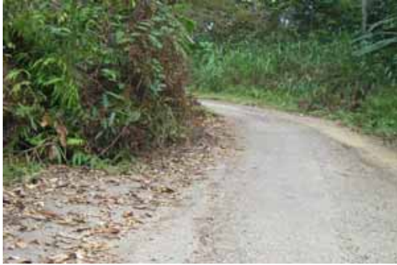
The bushes encroaching on the road
