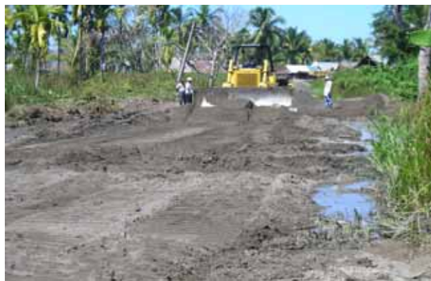
51 km north of Meulaboh there is a bad section at Arongan along 500 m. Infilling and grading has been started
