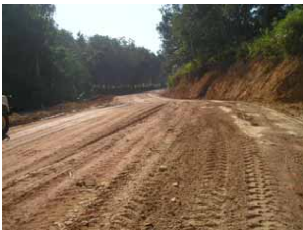
30 km north of Calang, a muddy section is in filled and graded
