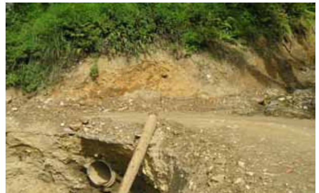
landslide, half of the road damaged but still passable
