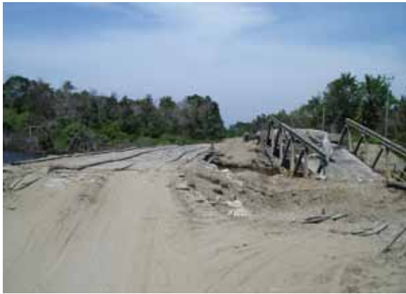
A wooden temporary bridge with a maximum capacity of 15 MT. The old bridge was damaged in the earthquake.
