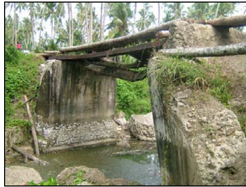
Broken bridge in Nias South of Sirombu
