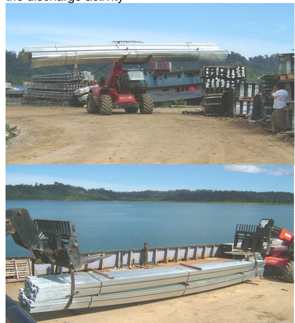
WFPSS Manitou forklifts assist cargo discharge from Daily Express I at Simeulue
